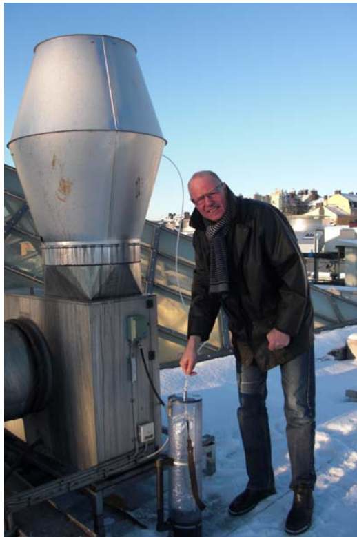
Figure 2 Odour sampling after the fan unit (sample point 6)
