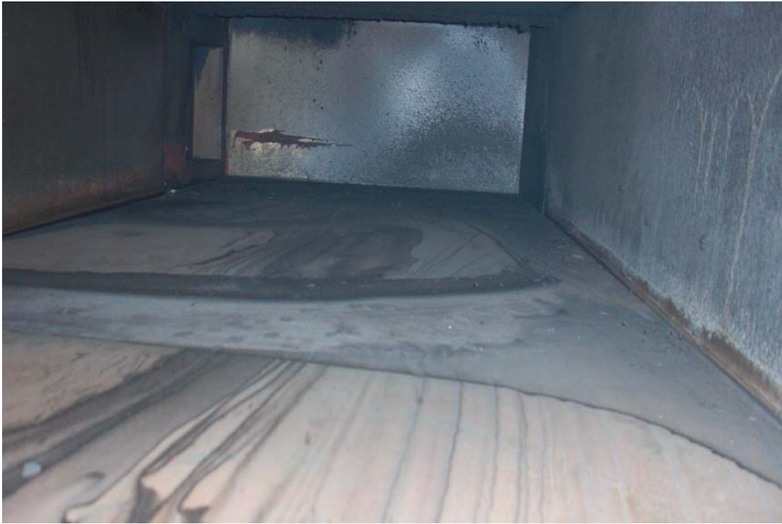
Figure 5 Picture inside the duct before installed AirMaid (December 2010).
